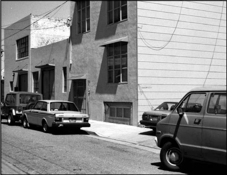
This building on Clara Street shows the effects of subsidence due to the thick soft sediments that underlie the South of Market area. The building has subsided several feet. The sidewalk and street have been built up to maintain the original grade level of the street. The top of the garage door is at waist level. The entrance door to the house has been repositioned to enter the house at mid-level. The window on the right was once on the second floor of the house.
